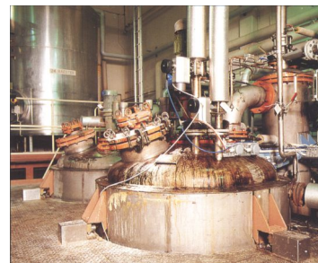
Batching Processes Reactors and Process Vessels
